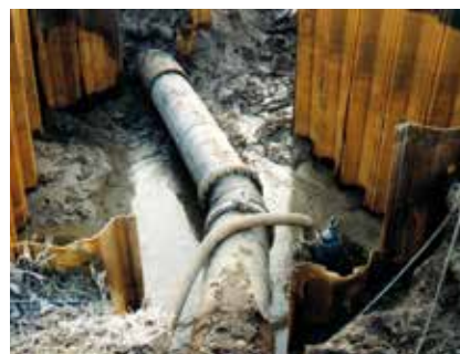
Existing cast iron pipelines
